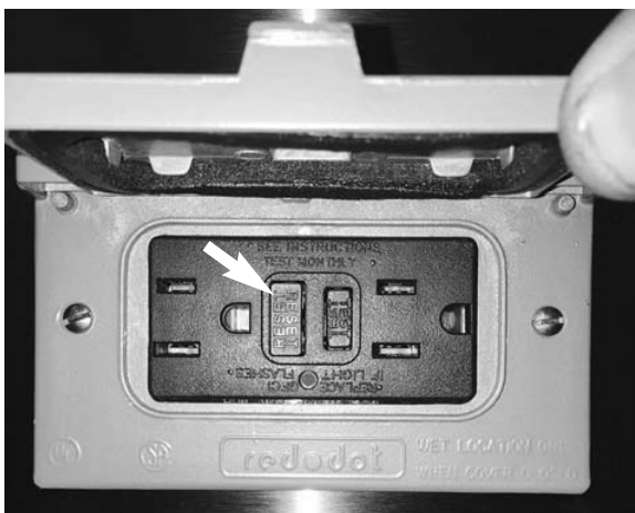
Figure 4-2. Reset Button on GFCI Outlet
