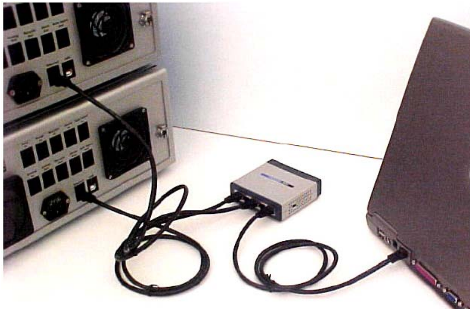
Figure E-17: Connecting multiple instruments to computer via Ethernet switch
